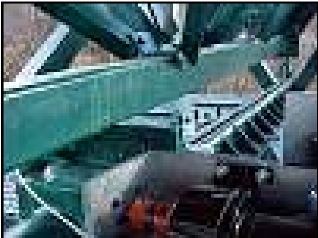
KL6M's broken dish el drive.
